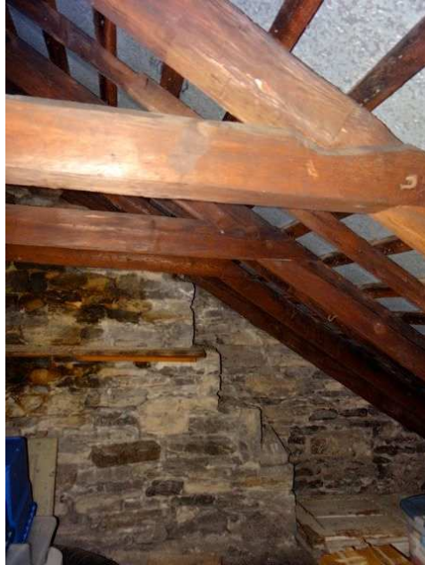
Notched beams in the attic of stone section; stone-enclosed flues against end wall.
